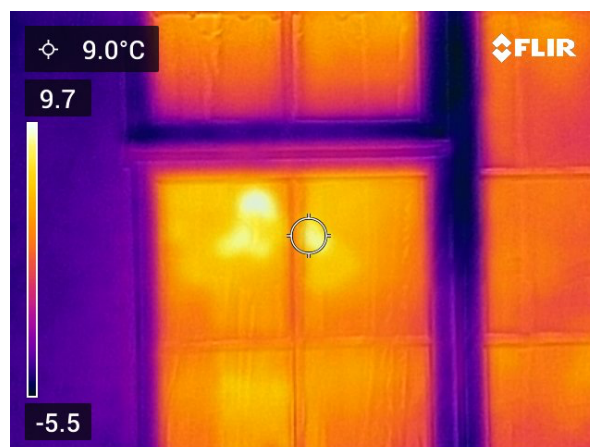
Single glazed window outside
